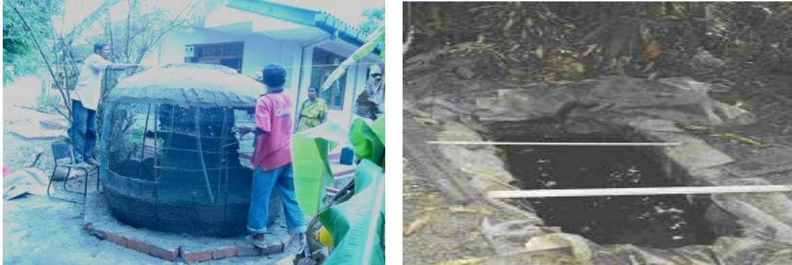
Figure 5a: Above the surface tank under construction (Credit: Janaki Chandimala) 5b: Polythene tank (Source: Moonasinghe V, 2004)
